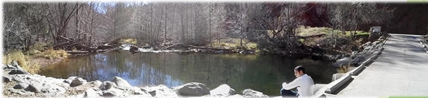
The scour hole downstream from the crossing
