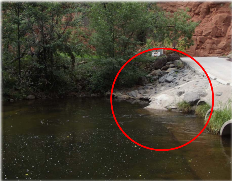
Scouring taking place downstream (notice the eroding concrete)
